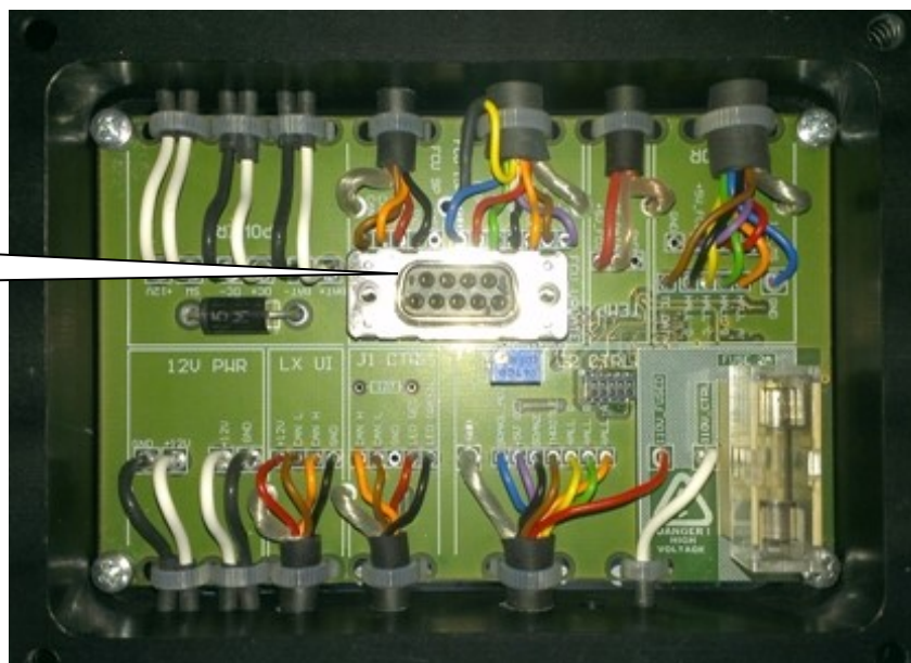
FCC (FES connecting circuit) with cover removed
