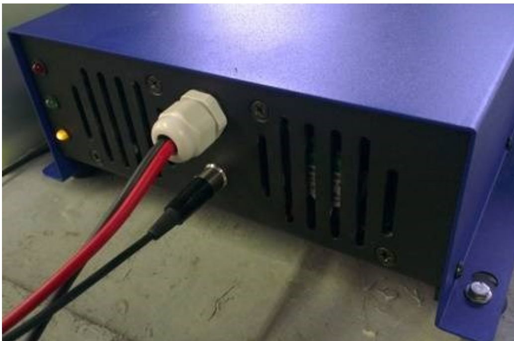
BMS-Charger signal cable plugged into the Charger; yellow LED light is ON-Charger is working
